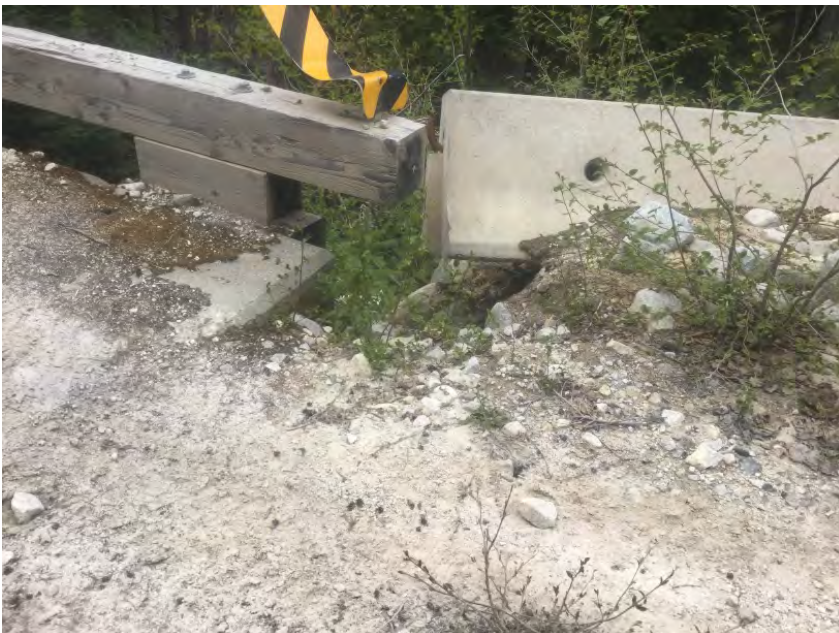
Loosing fill at downstream right approach
