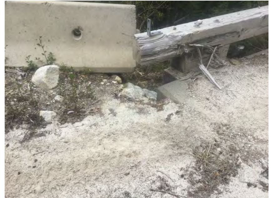
Loosing fill at downstream left approach
