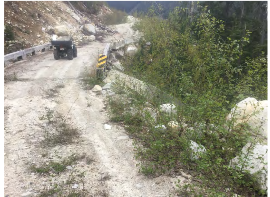
Failed no post barriers at downstream right approach
